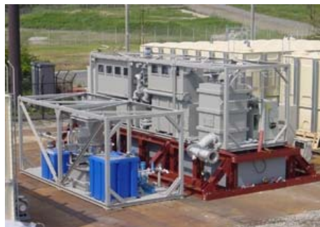
Ballast water treatment system
