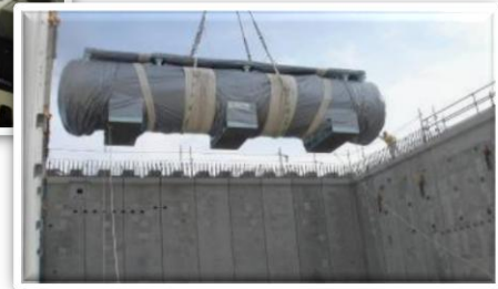
Radioactive waste storage facility equipment (sludge storage tank)
