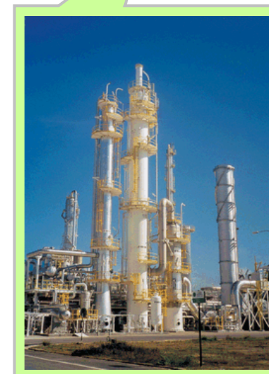
CO 2 capture plant designed for Malaysia Capacity: 200 tons/day
