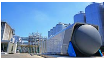
Biogas SOFC at Asahi Breweries Ibaraki Brewery
