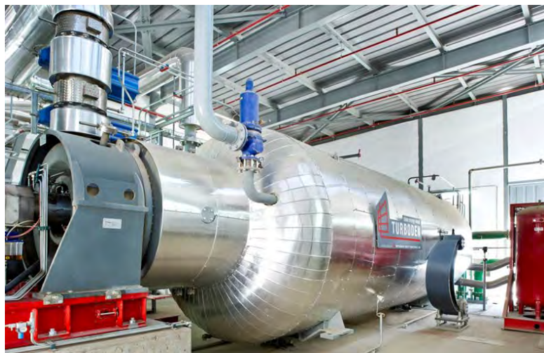
Turboden's Organic Rankine Cycle (ORC) power generation system
