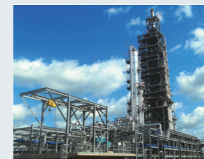
CO 2 capture plant
