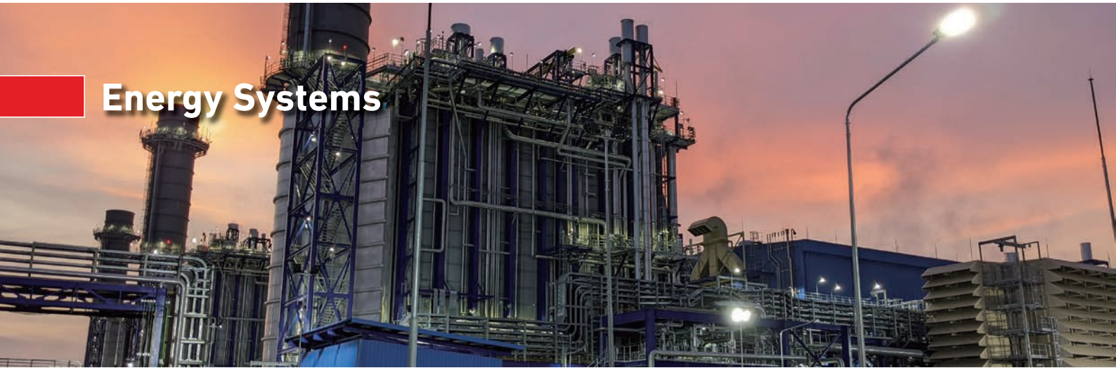
GTCC Power Plant (Thailand)
