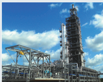
CO 2 capture plant
