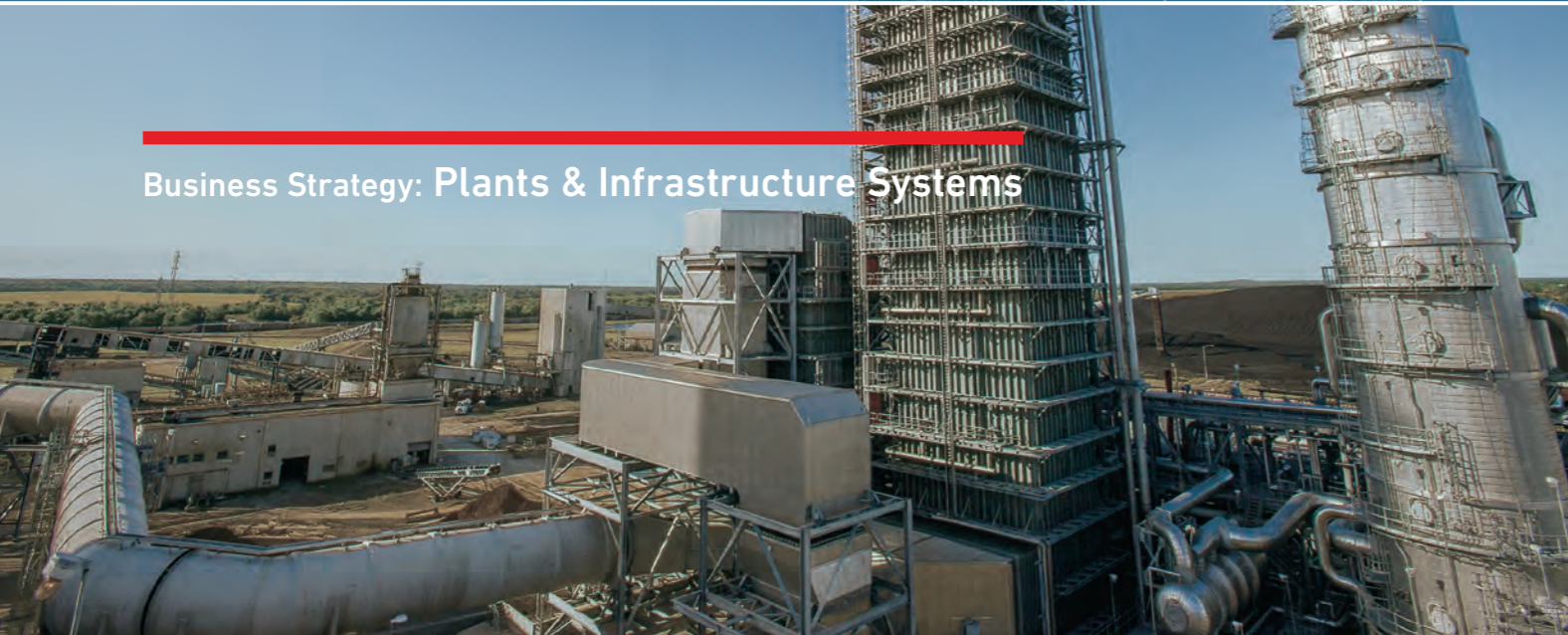
CO 2 Capture Plant (U.S.A.)
