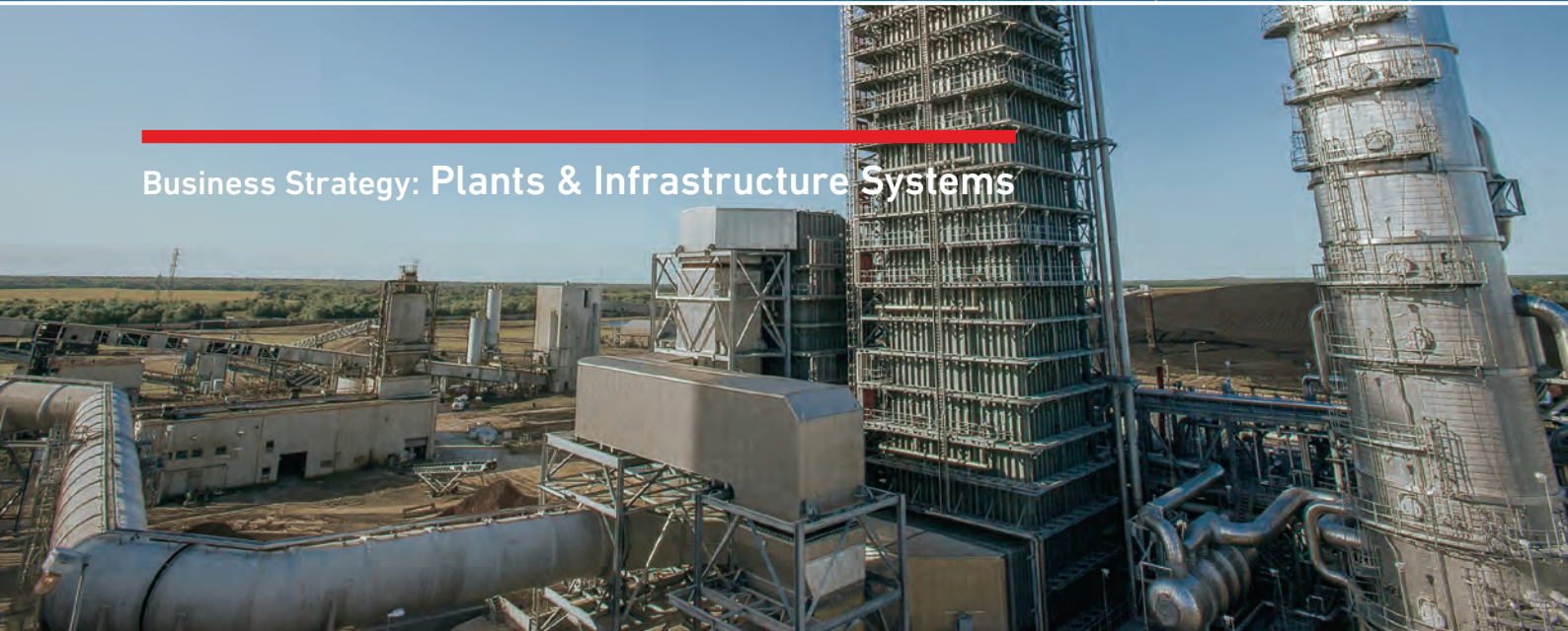
CO 2 Capture Plant (U.S.A.)
