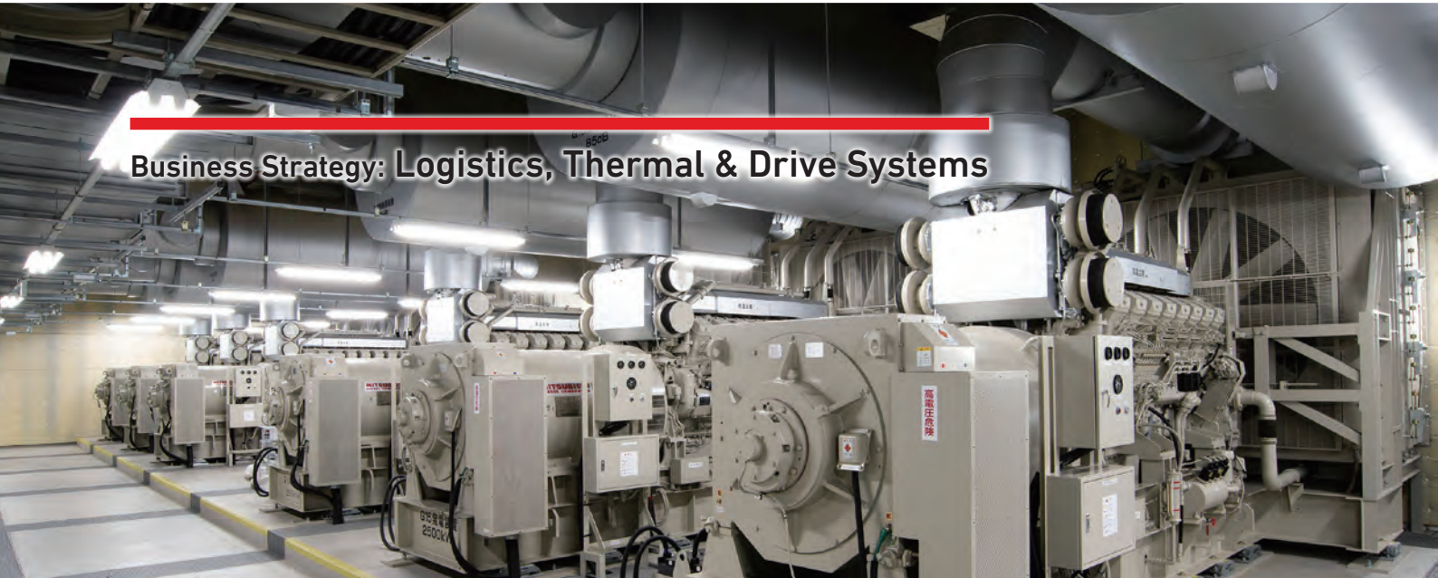
Engine Generator Sets for Data Centers
