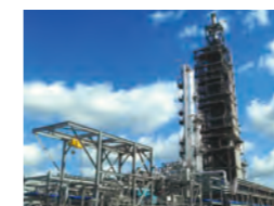
CO 2 capture plant
