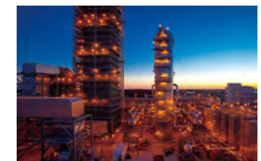
CO 2 capture plant (world's largest CO 2 capture volume of 4,776 tons / day for a power plant application)
