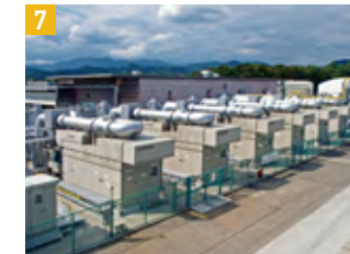
Highly Efficient Gas Engine Power Plant
