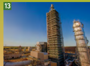
CO 2 Recovery Plant
