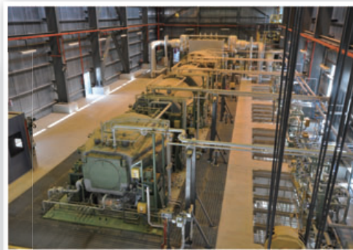
▲ Compressor and mechanical drive steam turbine for world's largest ethylene plant in the UAE
