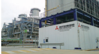
▲ EGAT Wang Noi GTCC Plant, Thailand
