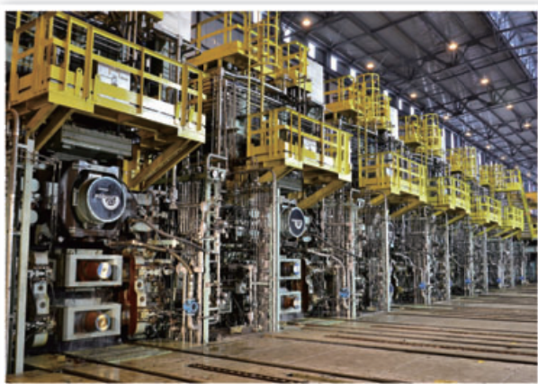
▲ Hot Rolling Mill
