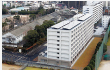
Solar cell panels installed at an MHI dormitory for single employees
