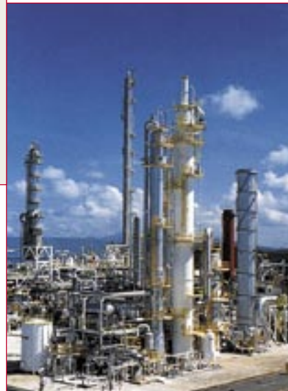
Flue Gas CO 2 Recovery Plants
